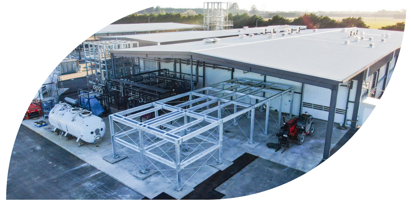
Complex Engineering - Tawhiri 1 Energy Hub
